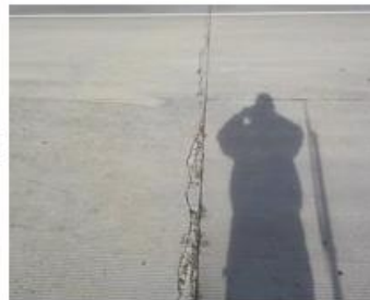
Near Approach Panel 2 Cracking
