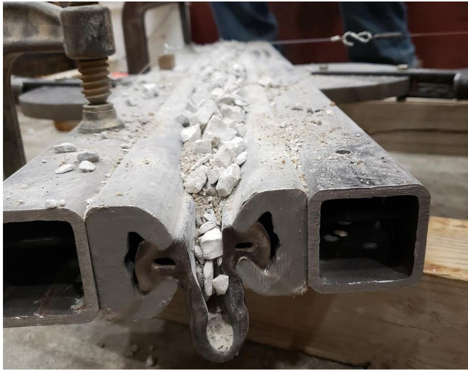
Figure 26: Restricted Closure Due to Debris (Typ.)
