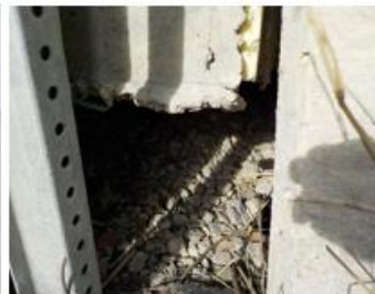
Erosion, thickness = 2 ft.
