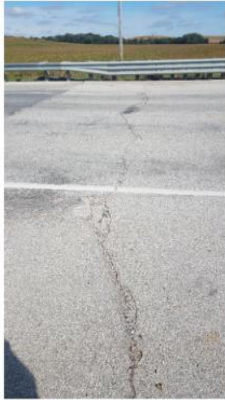
Figure 34: Transverse Cracking of Approach (Krapf, 2019)
