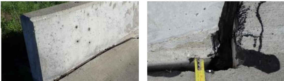
Figure 37: Examples of Voiding at Integral Abutment Bridges (IDOT)
