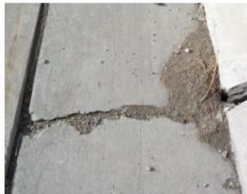
Far Approach Panel 1 Cracking
