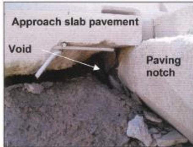
Figure 30: Voiding Under Approach Slab (White, 2007)
