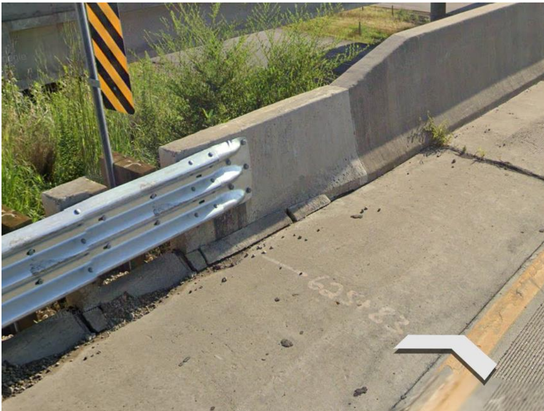
Figure 40: Cracking at Barrier Rail Indicating Settlement
