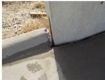
Barrier Diff Settlement/Cause of Drainage
