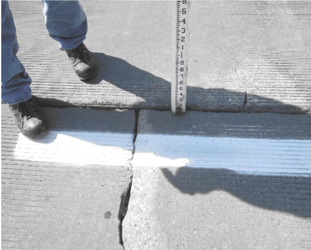
Figure 41: Differences in Slab Height Indicating Settlement
