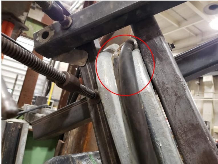
Figure 12: Closure Limit Due to Sealant Bending
