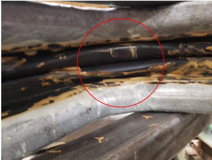
Figure 21: Upturned Section Unable to Completely Close
